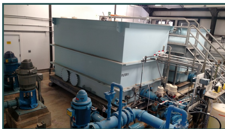
Water District 19 Water Treatment Plant
